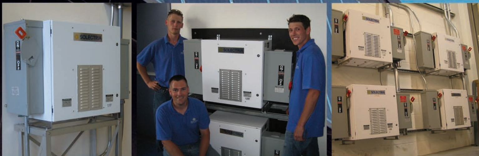
Background & Left: 13.8 kW system at Evergreen Solar's mfg. facility Center: 35 kW NexAmp installation at Ebsco Publishing Right: 120 kW system (4 of 8 inverters) by Chico Elec/Solar Design Assoc, AT&T Park, Giant's baseball stadium, San Fran, CA
